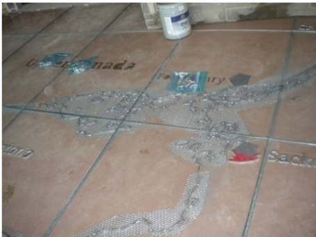
3D letters and the outlines of the map are in position before the terrazzo are poured in
